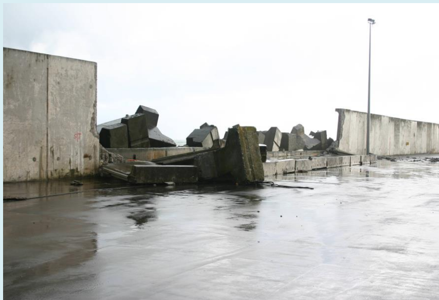
Storm damage, Port of Taranaki, New Zealand. Photo courtesy of Peter Atkinson
