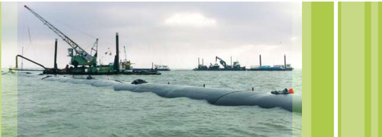
Pontoon with crane filling the 'zandworst' in the foreground with a sand-water mixture transported and produced by the installation on the background.
