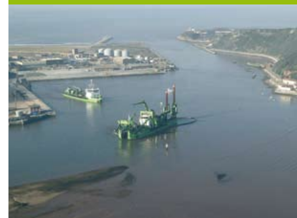
Deepening of the access channel to the port of Aviles in Northern Spain. These rock dredging works involved the combined intervention of a brand new seagoing rock cutter dredger "D'Artagnan" with trailing suction hopper dredger "Antigoon".
