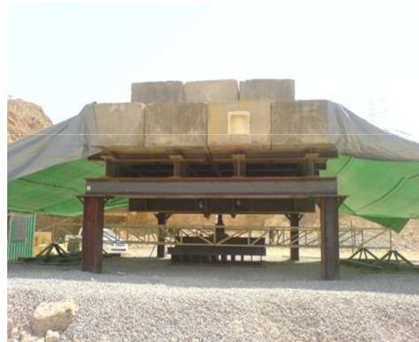
Load test applied to quarry run bund of 9m height 160 kPa load for 3 weeks, increased to 210kPa
