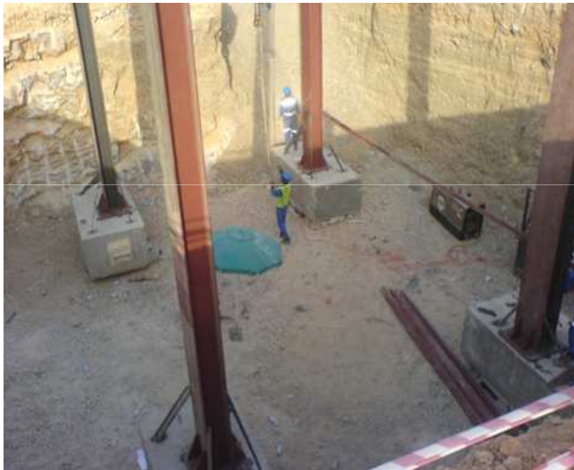
Excavated pit for test setup on settlement of quarry run foundation under quaywall
